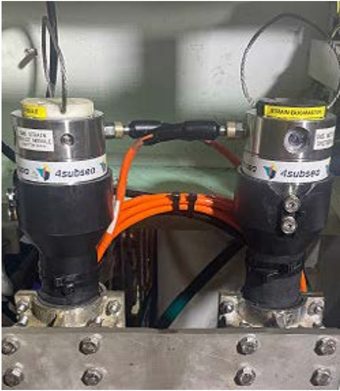
Offshore deployment of SMS Strain™
